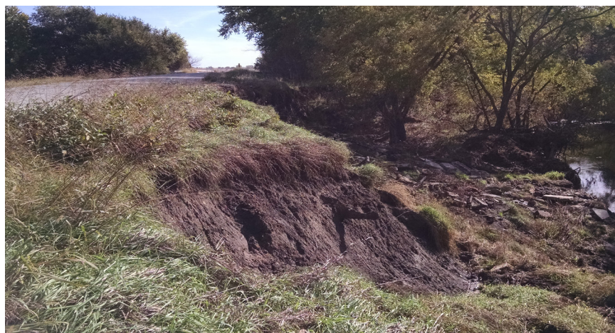
Brown County EWP exigency streambank stabilization. High traffic county roadway impacted by flooding.
